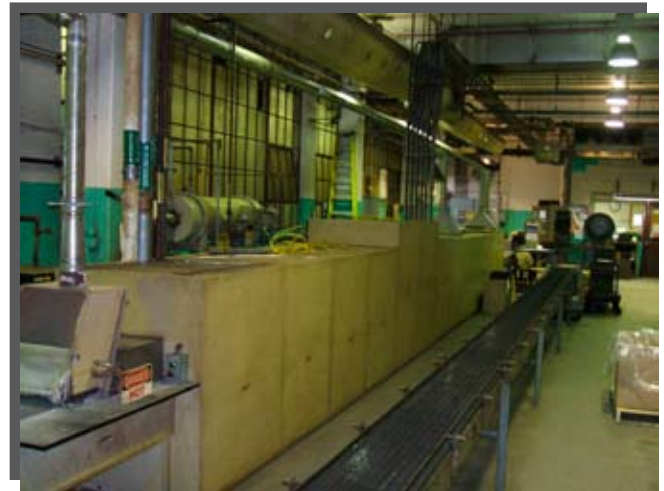
The annealing furnace at National Rivet & Manufacturing Company comprises 24 separate electric heating elements—with temperatures reaching as high as 1650 degrees F—all controlled by a Trend IQ3 system with pinpoint accuracy.
